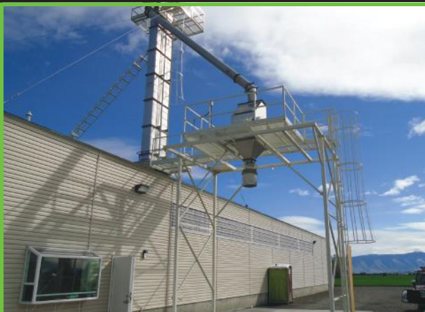
Product conditioner in load out.
